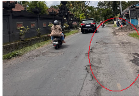
Figure 6. Potholes and uneven road surface
