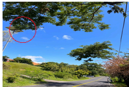
Figure 5. Street lights are obstructed by vegetation.
