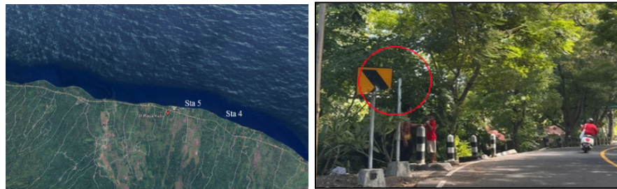
Figure 4. a) The Kubu Tejakula road segment. b) damaged traffic signs
